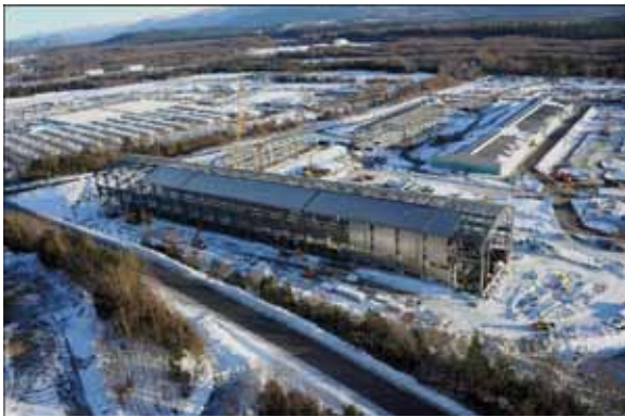
Aerial view of the Kitimat Modernization Project site. Photo courtesy of RTA/Bechtel
