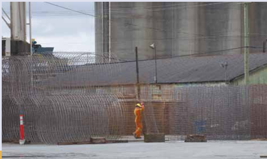
"We do giant underground plumbing here," said Yves Guimond, superintendent at Ocean Pipe in south Vancouver. "Only the worms will see it [but] this is the foundation of every prosperous city." This steel from Tree Island Steel (a Teamsters' signatory) will be used to reinforce the concrete storm and sewer pipes found under many B.C. communities.
