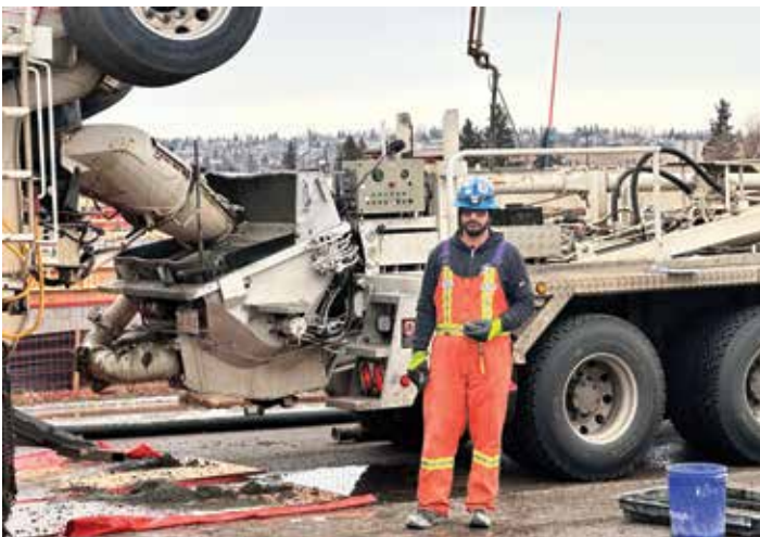
Harpal Singh, mixer driver at Heidelberg Concrete Dawson Creek, feeding the pump truck at the Dawson Creek Hospital site.
